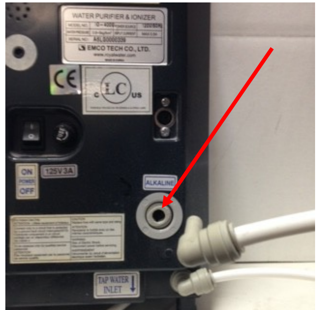
Alkaline Water Outlet With 5/16" Tubing Disconnected Mineral Buildup will appear here and will look like previous photos
